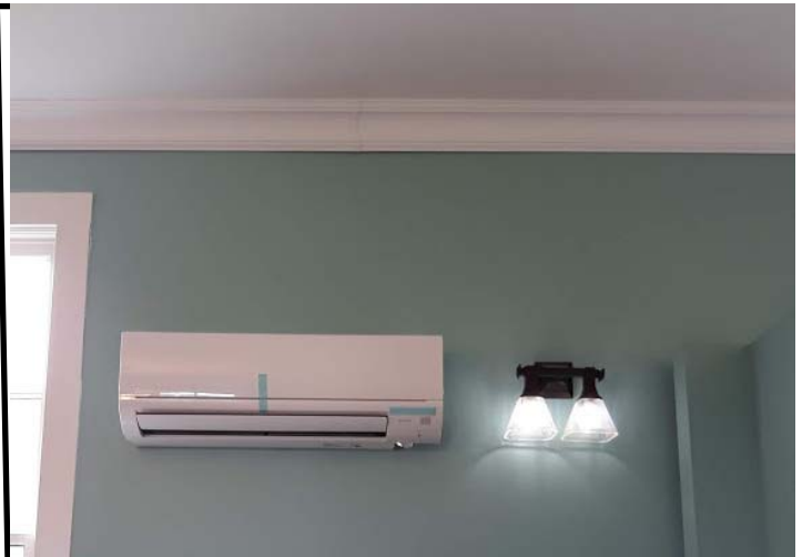
Ductless Heating Unit
