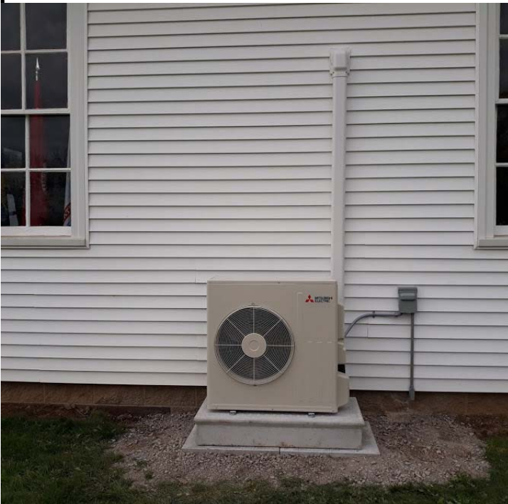
Air Conditioner out side the Treichler Building
